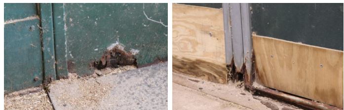
The new mesh stalls (top) vs. the corroded, outdated stalls (bottom).
